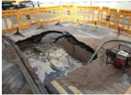
Figure 5: Road collapse caused by Water Main Burst (Fenland Citizen, 2012)
