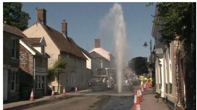
Figure 4: Burst Water Main (BBC, 2010)
