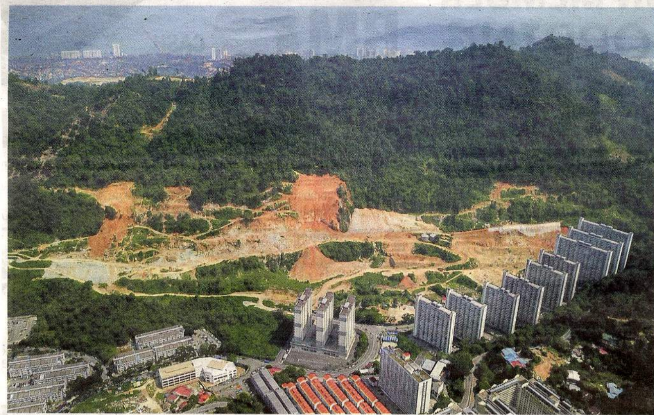
Bare hills: An aerial view of the hill clearing taking place near Majestic Heights (bottom right of pic) in Paya Terubong area. — ZAINUDIN AHAD/The Star
