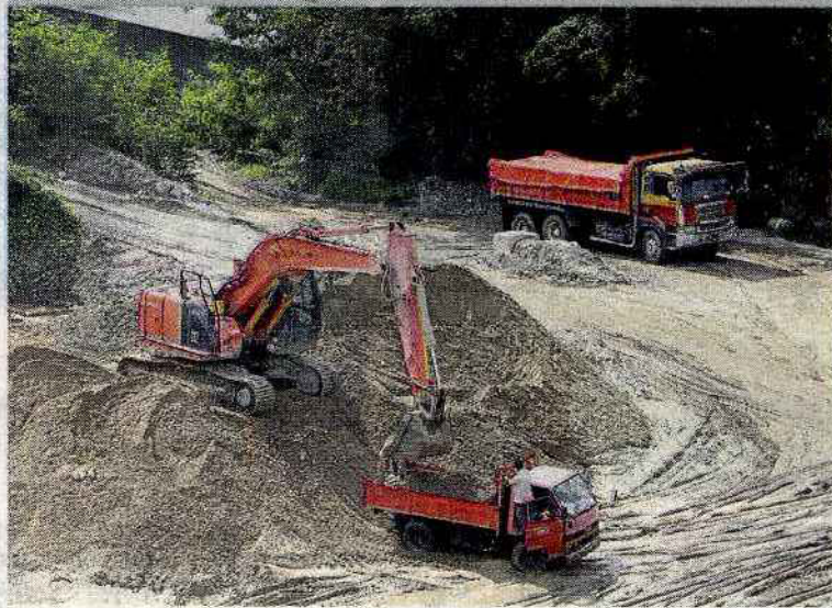
Trees and hoarding surround the site, making it impossible to see the activities from ground level.
