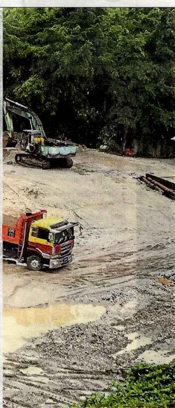
An excavator scooping up sand into 10-tonne tipper lorries that transport the sand out of the area. — Photos: YAP CHEE HONG/ The Star
