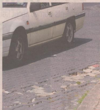
Bad job: Badly-paved roads are a common sight in PJ.
