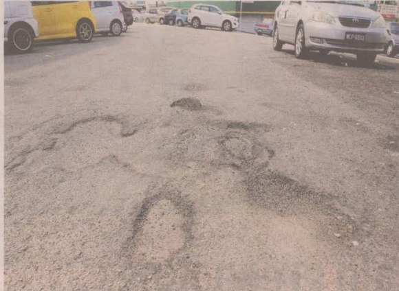
Bumpy ride: The terrible road condition near Jalan 21/17 in Seapark.
